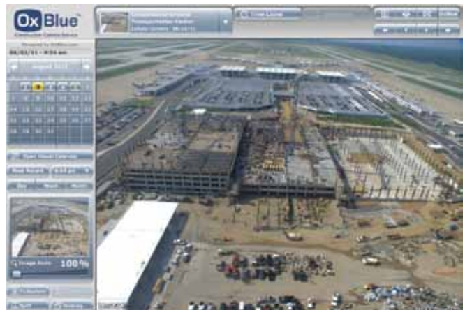
One of the ways Flintco, LLC Project Manager, Tony Caldwell uses the OxBlue camera on this Memphis International Airport jobsite is to review recent historical data to make immediate changes in real time to keep pace with the current situation.
