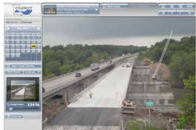
Traffic disruption was limited to 20 days. Adhering to the aggressive timeline was made easier with an OxBlue camera.
