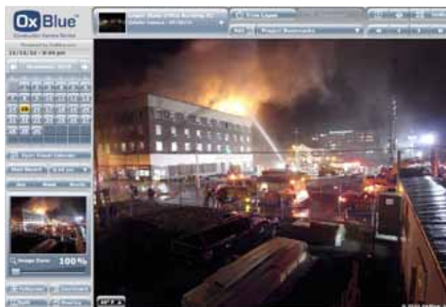
OxBlue’s high-resolution, time-lapse construction cameras allowed Massaro Corp. to fully document building-site damage caused by a nearby fire.
